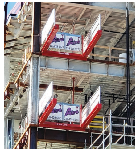
A photo of two Generation 1 LTDs in place shows the concept of the transfer deck system.
